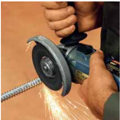
3. Cut threaded bar to exactly the required length using metal saw or right-angle grinder.
